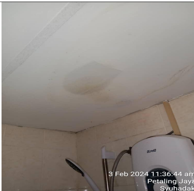
Picture 3: The ceiling and water mark on the wall located at master bedroom toilet area.
