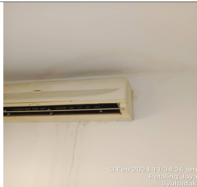
Picture 4: The damages ceiling and water mark located at room 1 area.
