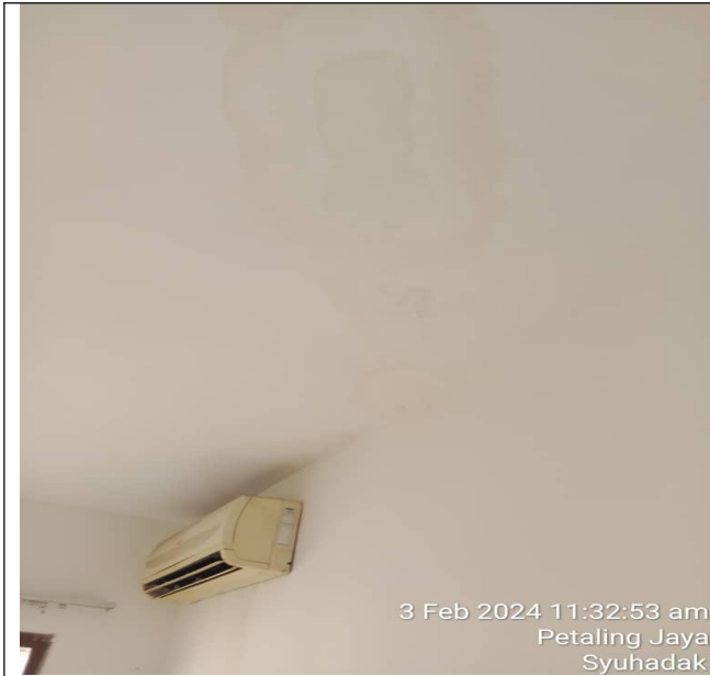
Picture 1: The damages ceiling and water mark located at room 1 area.
