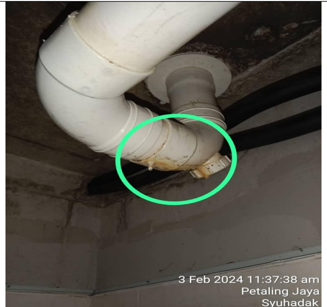
Picture 2: The water mark suspect due to the pipe leaked at master bedroom toilet.
